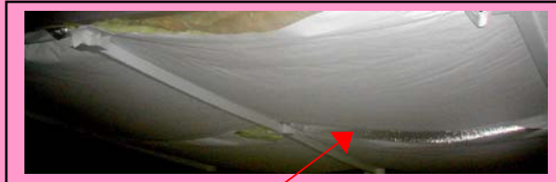
Facing tabs are pulled out, Plastic Extrusions installed parallel and under purlins.
